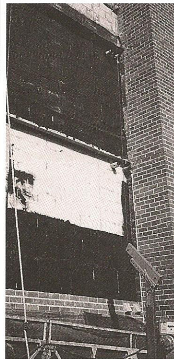
Damage within building façade required new waterproofing systems
