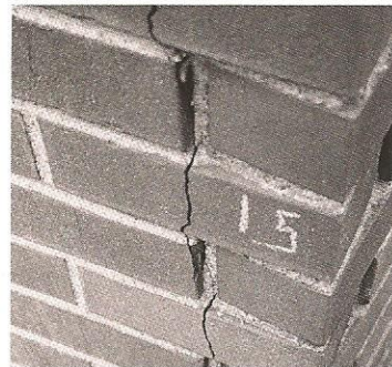
1/2" crack in brick veneer required repair
